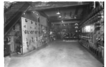
AFC 341-S4-SS1-I22 Horton Street Station - switchboard floor. -- 1912. -- 6.5x8.5 copy of glass plate negative. -- Box Number AFC 341-18
