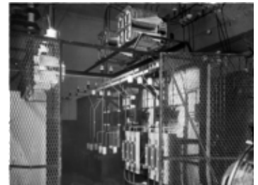
AFC 341-S4-SS1-I20 Horton Street Station - equipment 3. -- 1912. -- 6.5x8.5 glass plate negative. -- Box Number AFC 341-4 AFC 341-18
