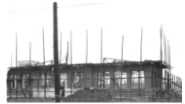
AFC 341-S6-I19 Building renovation 3. -- [between 1907-1928]. -- 8x10 glass plate negative. -- Box Number AFC 341-10 AFC 341-19
