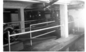
AFC 341-S4-SS1-I24 Horton Street Station - generators 2. -- 1912. -- 6.5x8.5 glass plate negative. -- Box Number AFC 341-4 AFC 341-18
